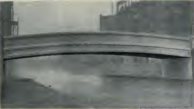
An Artistic Concrete Bridge with Simple yet Graceful Lines—A Direct Contrast to Many of our Highway Bridges.
